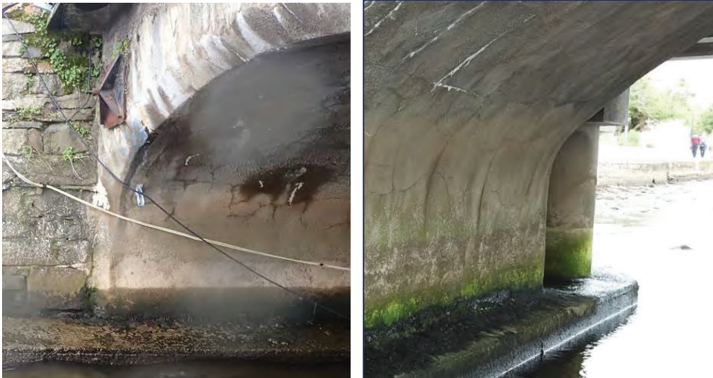
Figure 4.6: Examples of Gunite Areas Requiring Repair
