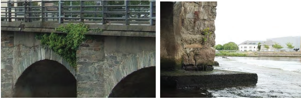
Figure 4.7: Vegetation Growing on Bridge
