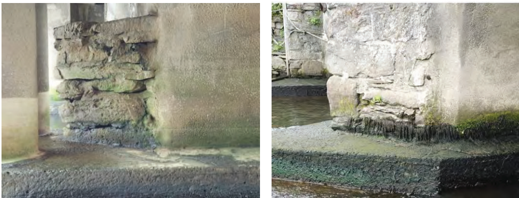
Figure 4.8: Examples of Masonry Requiring Repair
